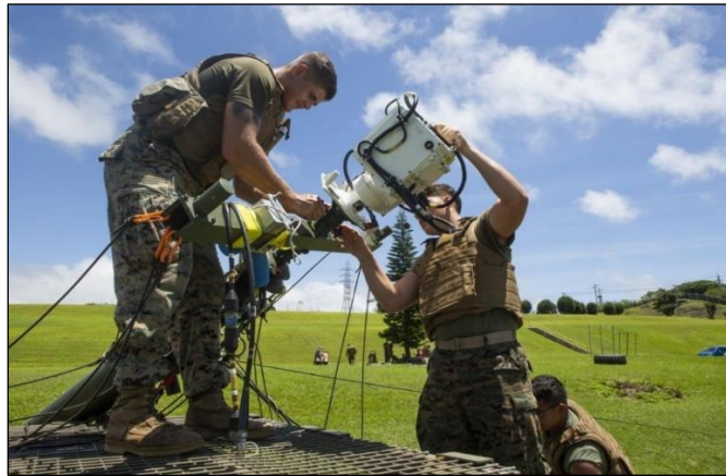
Figure 7. U.S. Marine Corps Free Space Optics Communications System
